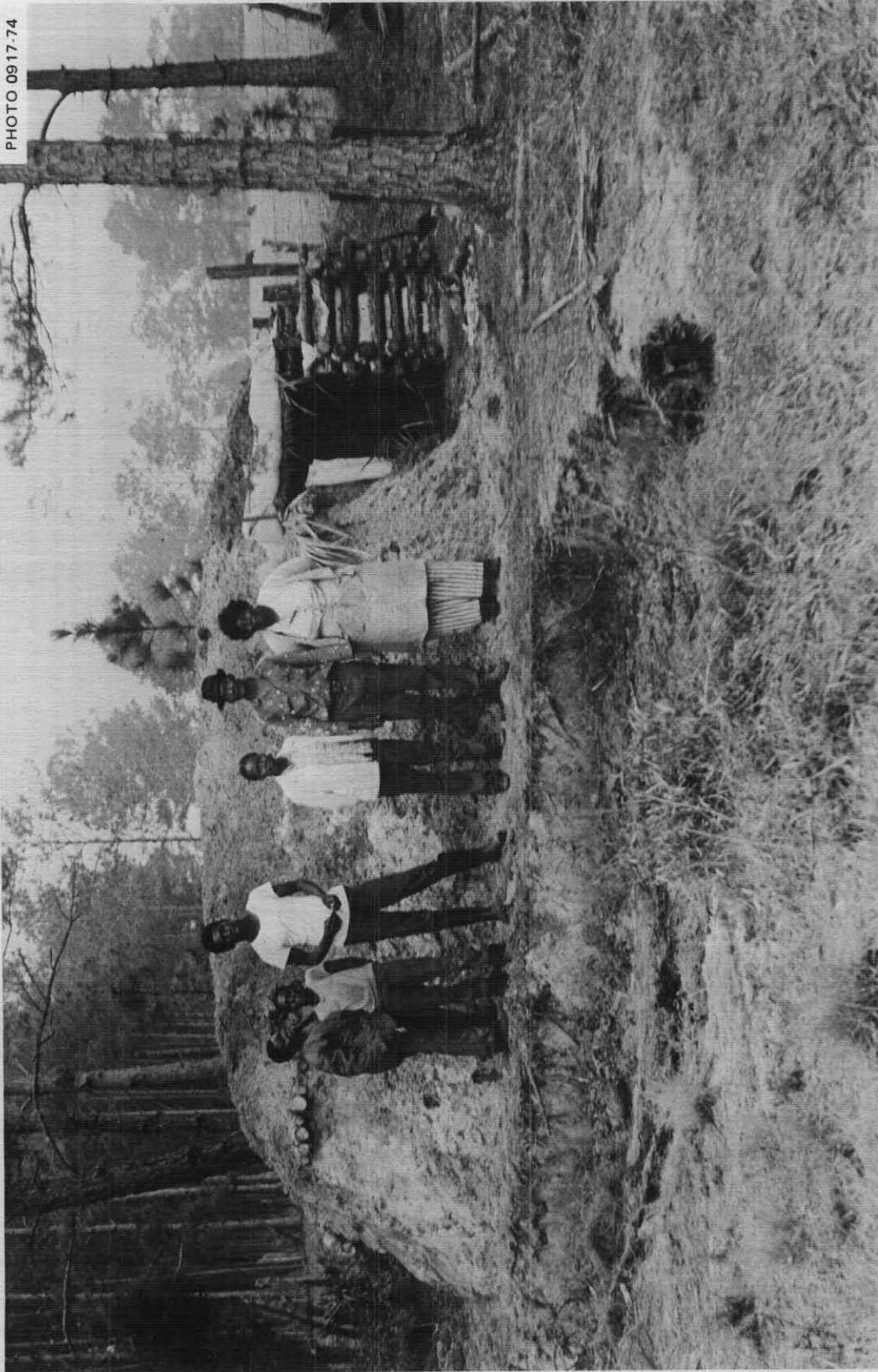
Fig. 5.24. The successful builders outside their completed shelter, with a full 2 ft of earth on the roof. Note one of the shallow barrow pits, from which they had shoveled and carried earth, in buckets and a wheelbarrow, to the adjacent building site.
